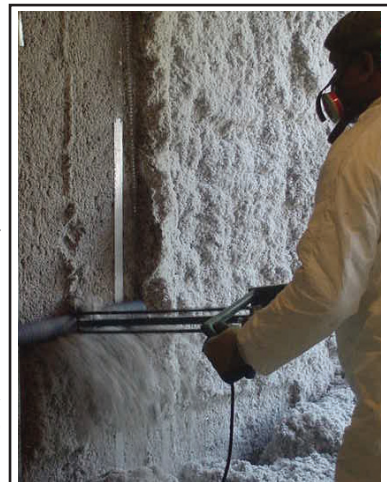
INSTALLATION includes scraping down the damp-sprayed papier maché like material for a flush to the stud finish. (All photos provided by Community Environmental Center)
